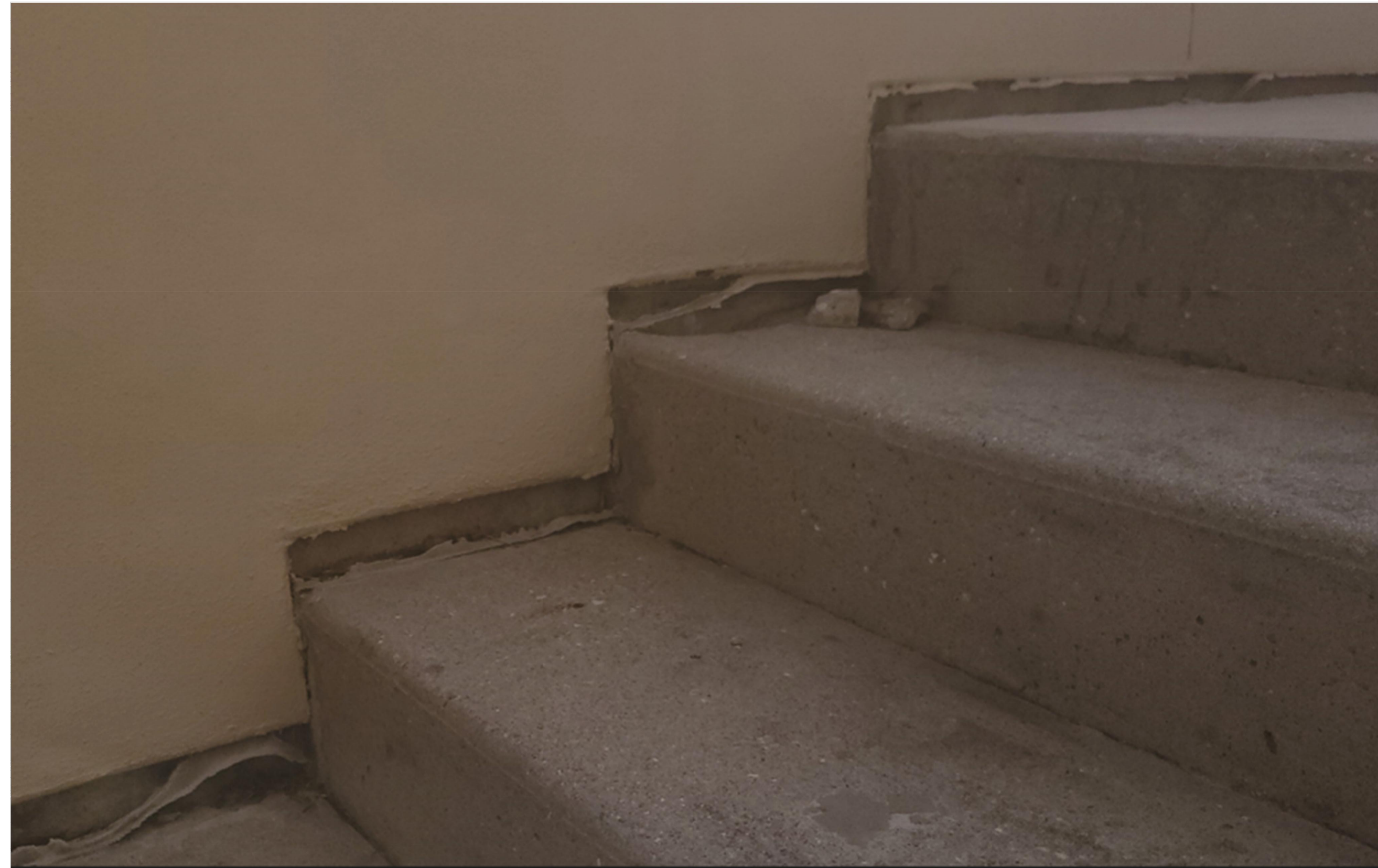
EAST SIDE OF STEPS, SHOWING SETTLEMENT AND VERTICAL DISPLACMENT FROM WALL
