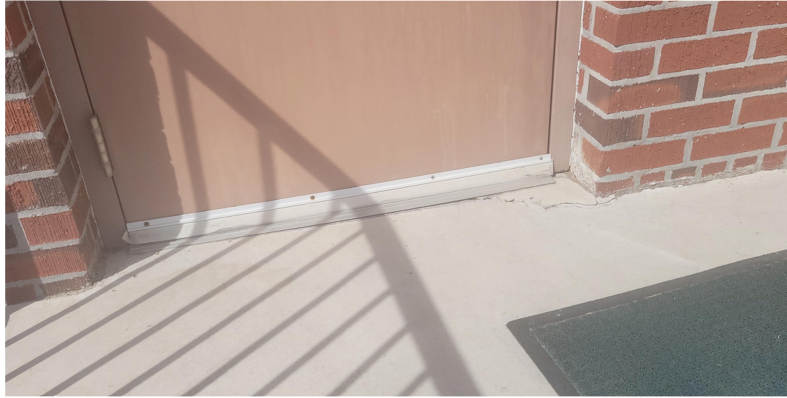
WEST SIDE OF TOP SLAB, NEAR DOOR TO COURTHOUSE. NO LARGE SETTLEMENT VISIBLE, ONLY A SMALL SPALL AREA
