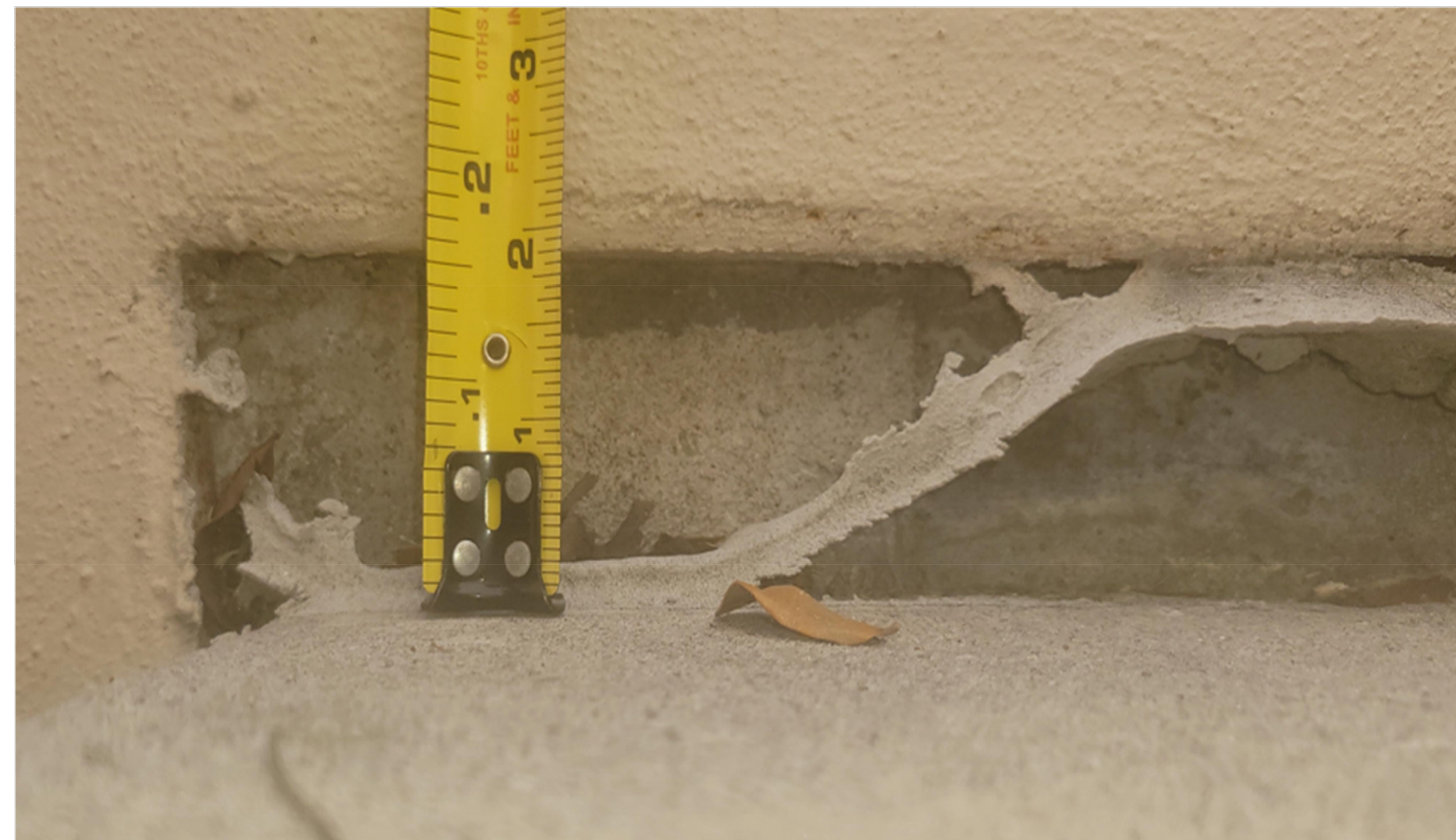
DEPTH OF VERTICAL DISPLACMENT AT STEP / WALL INTERFACE VARIES AND IS AS LARGE AS 2.2 INCHES
