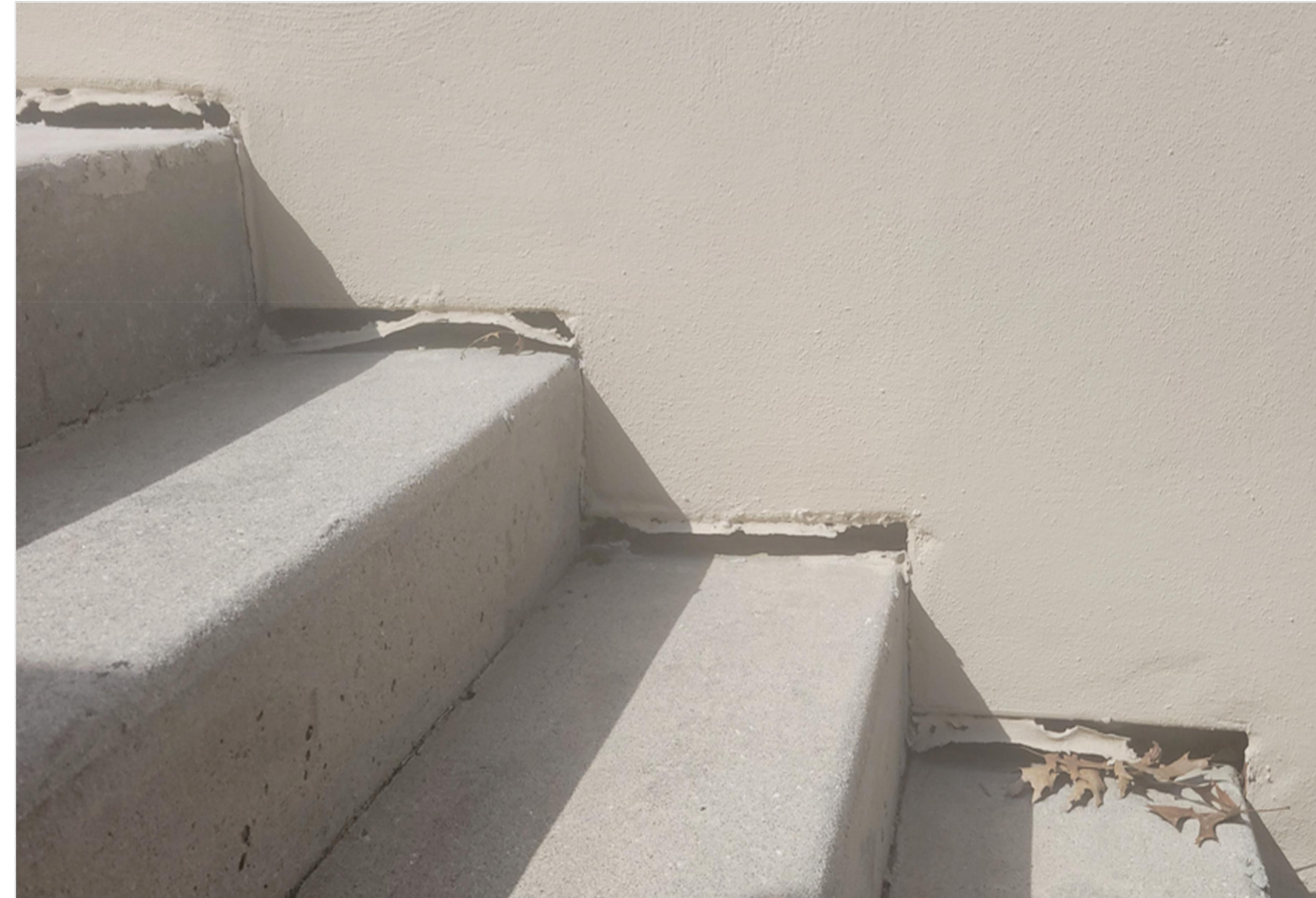
WEST SIDE OF STEPS, SHOWING SETTLEMENT AND VERTICAL DISPLACMENT FROM WALL
