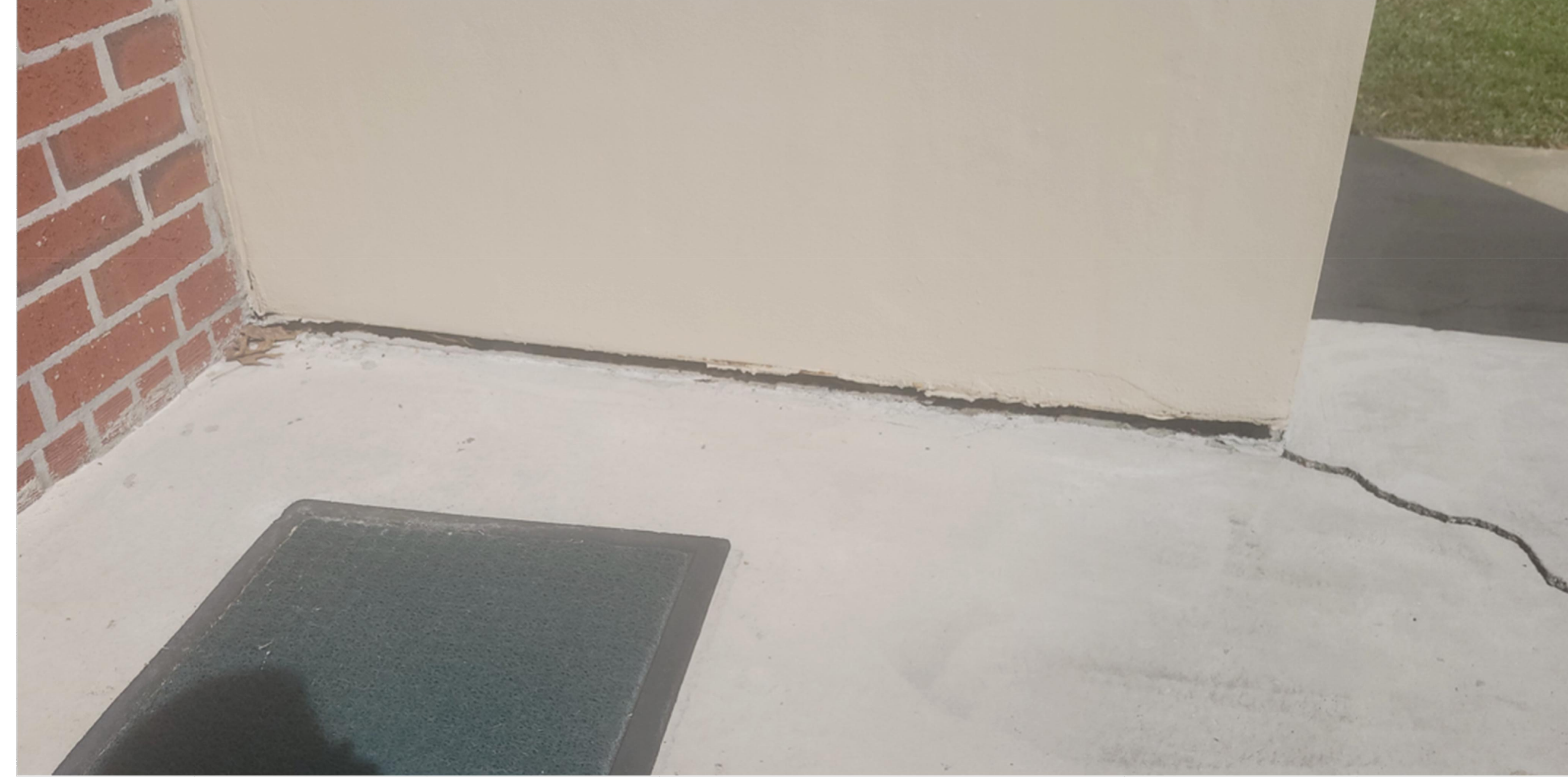
NORTH SIDE OF TOP SLAB. LARGE CRACK IN SLAB AND VERTICAL DISPLACEMENT FROM WALL.
