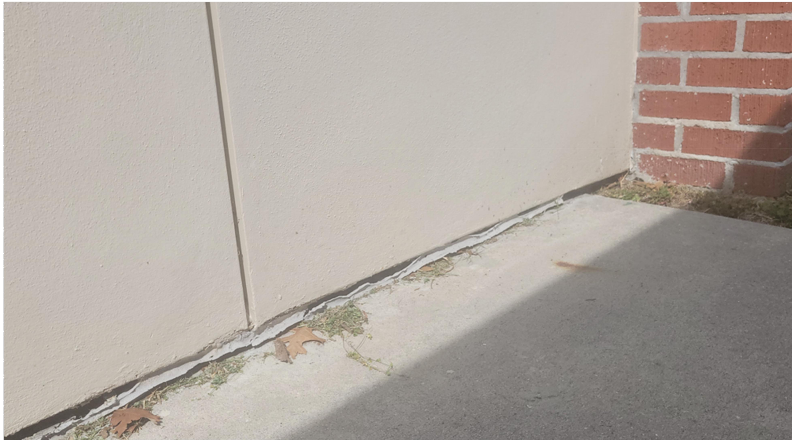
VERTICAL DISPLACEMENT AT BOTTOM SLAB AND COURTHOUSE WALL, WEST SIDE.
